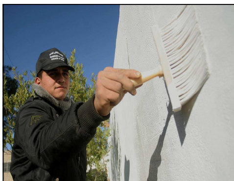
Giving school walls a first coat of paint, before the murals take shape.
